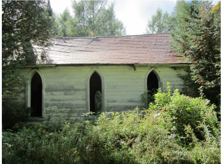
IN 2012, ST. MARY'S ANGLICAN CHURCH WAS IN AN ADVANCED STATE OF DETERIORATION (GSLR-27-1).
